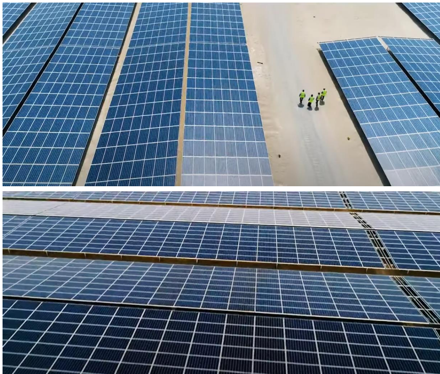
JinkoSolar 1177MW Abu Dhabi Solar Power Plant Abu Dhabi near Al Ain
